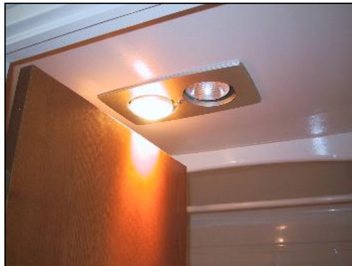
8. Heat lamp over door - fire hazard!
