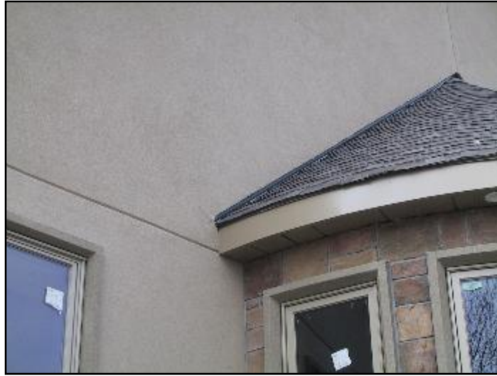
1. No kickout flashing at roof/sidewall junction
