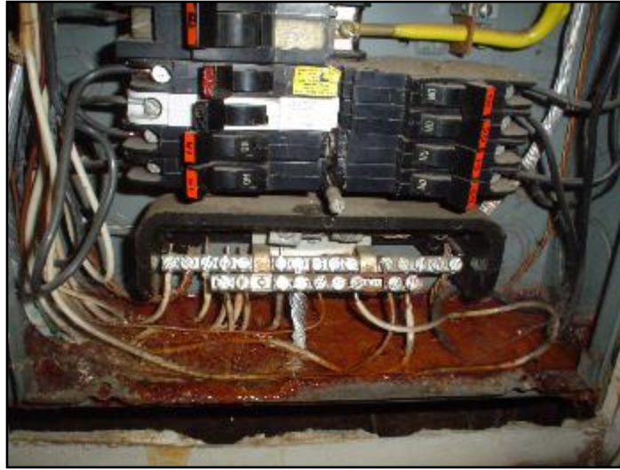
6. Water and rust in bottom of panel
