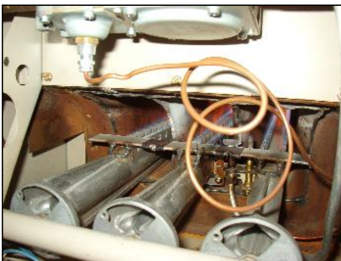
9. Rust at bottom of heat exchanger
