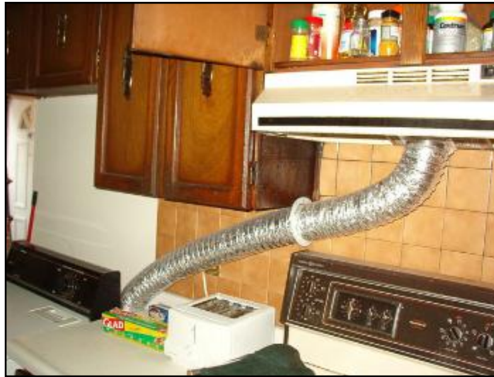
22. Clothes dryer vented incorrectly
