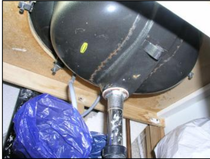
19. Steel basin rusting at weld
