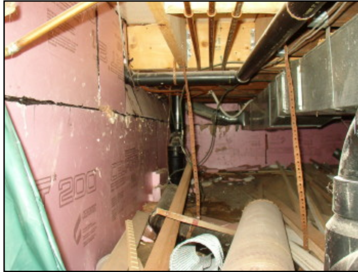
15. Exposed polystyrene insulation is fire hazard
