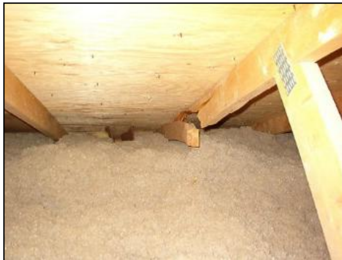
5. Top chord of truss is broken
