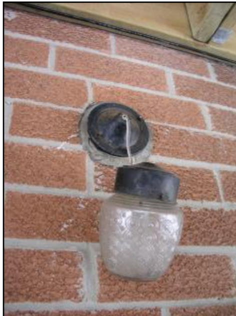
7. Light fixture is not well secured
