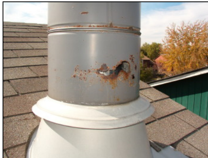
13. Rusted chimney wall from fireplace
