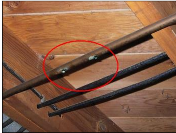
16. Leaking copper supply pipe
