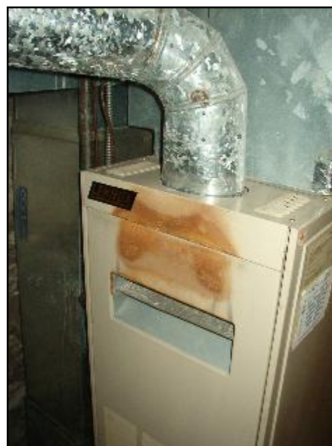
10. Evidence of furnace backdrafting
