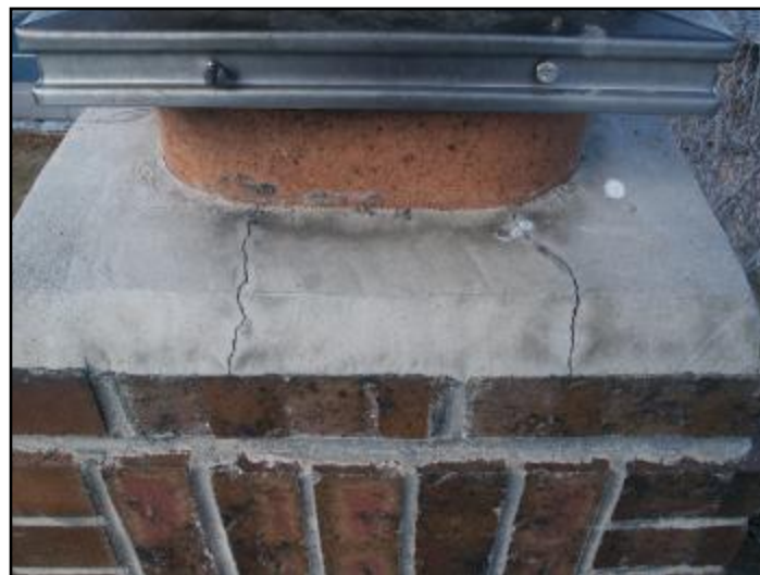
12. Minor cracks in chimney cap
