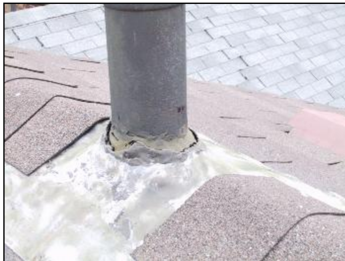
2. Stack flashing should be sealed.
