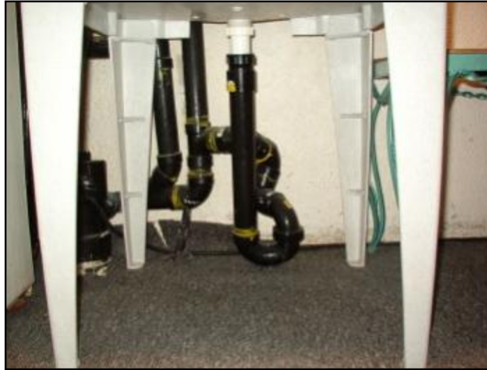
17. Poor trap arrangement
