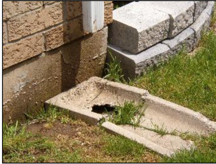
3. Downspout should be extended away from home
