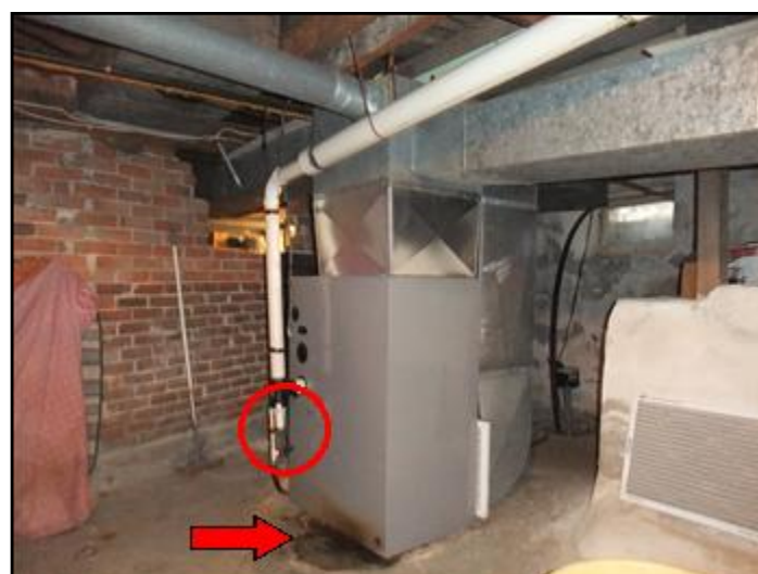
20. Leaking condensate drain
