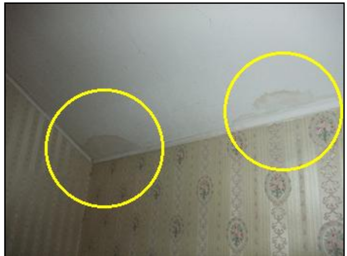
25. Stains below eaves, possibly from ice dams
