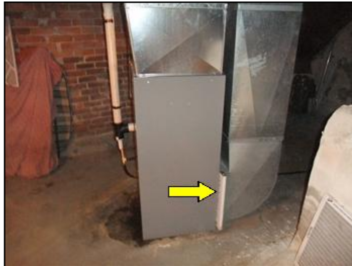
19. Rear view of hi-eff furnace, filter location
