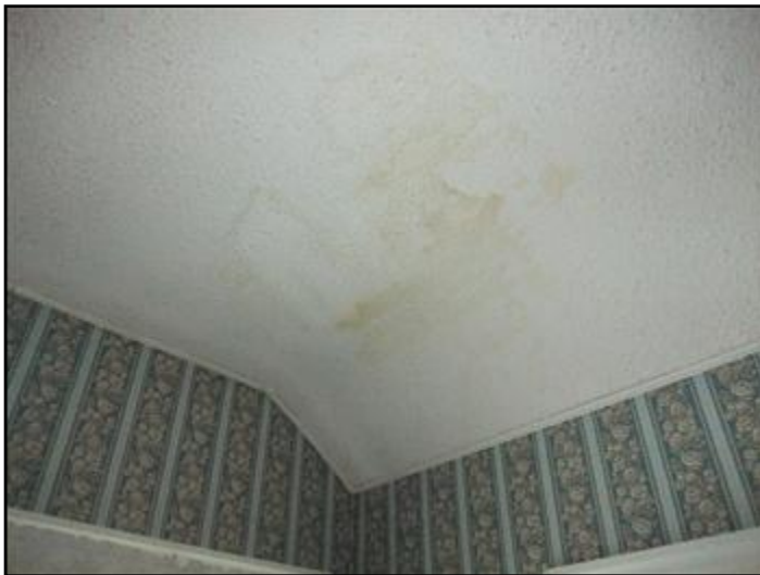
22. Appears to be a paint problem
