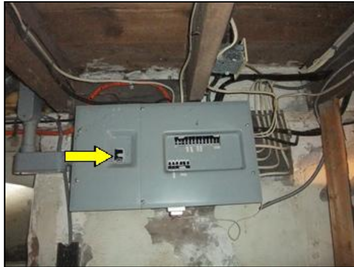
13. Distribution panel, main shut-off
