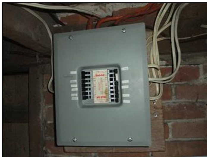
14. Sub-panel located in furnace room
