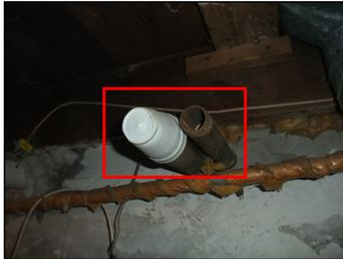
21. Abandoned fuel oil pipes
