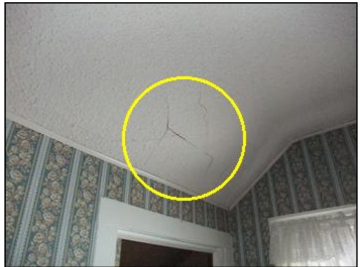
23. Loose, cracked plaster/lath
