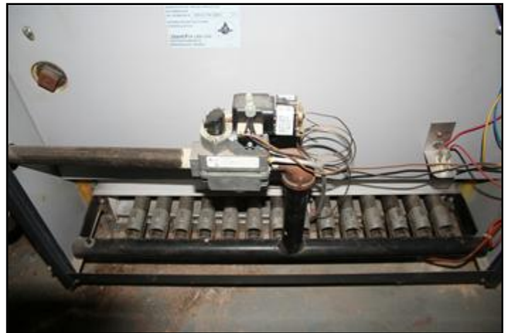
4. Front of burners
