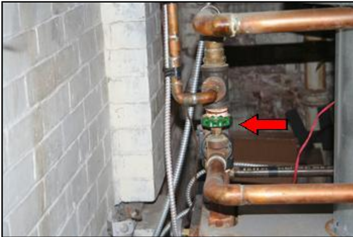
9. Suspect manual valve on bypass loop
