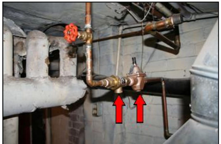
18. Backflow preventer and water make-up
