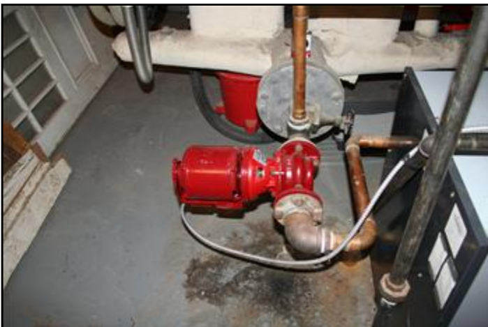
17. Circulator on return side
