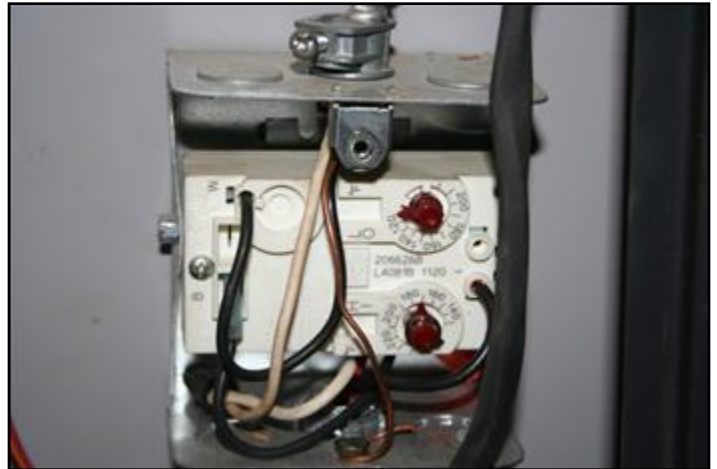
14. Pump control and high limit switch
