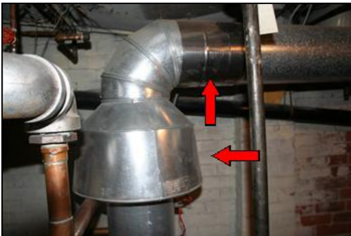
11. Draft hood - auto vent damper is above
