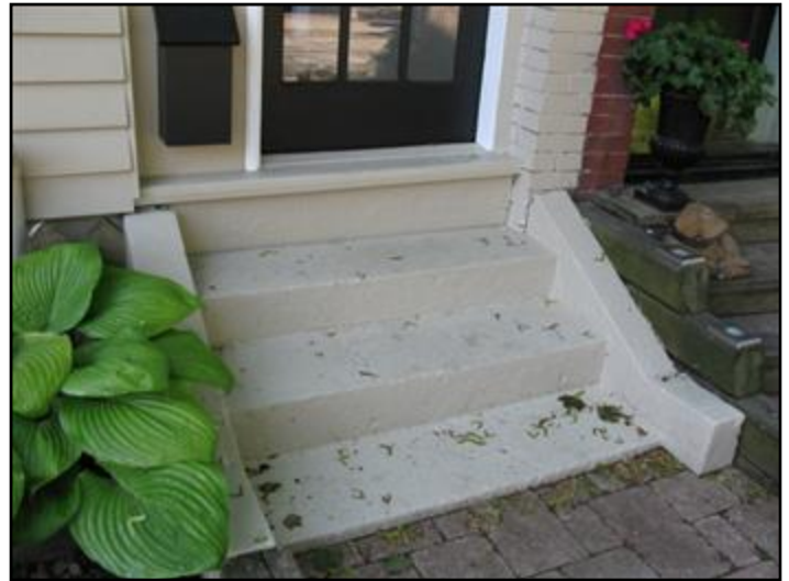
8. Front steps - no handrail
