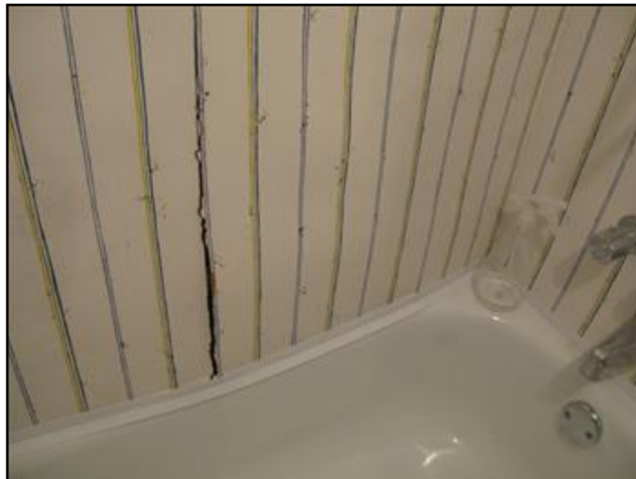
16. Low-quality, wood tub enclosure
