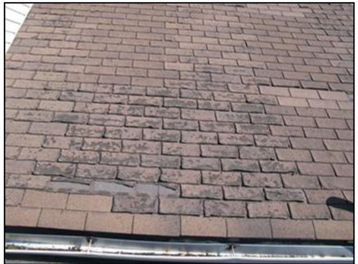
4. Worn out shingles
