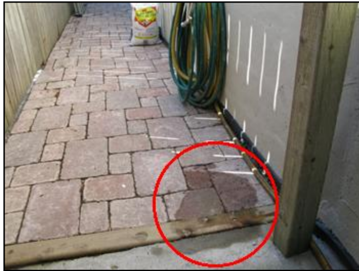
9. Poor slope for drainage
