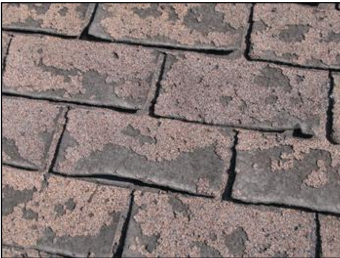
3. Closeup of worn out shingles
